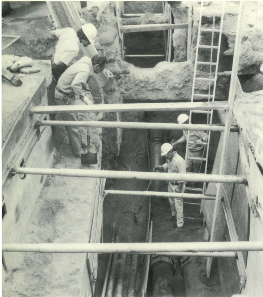
ABOVE: To provide clearance for a new Pasadena city storm drain, the Plant Maintenance staff excavates and lowers 14 underground conduits containing much of the College's communication lines and chill water ducts.
